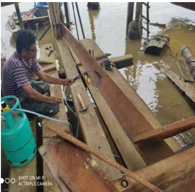
Figure 8: Process of Parching using Gas Fire
