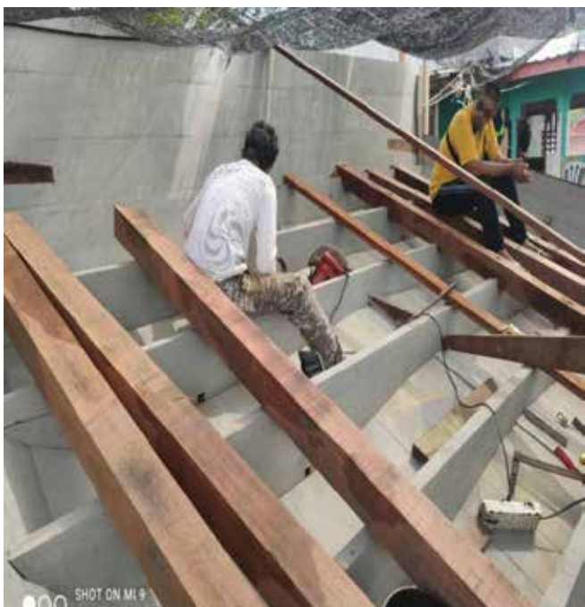
Figure 15: Installation of the Poop Deck's Frames to the Rear Part of a Boat
