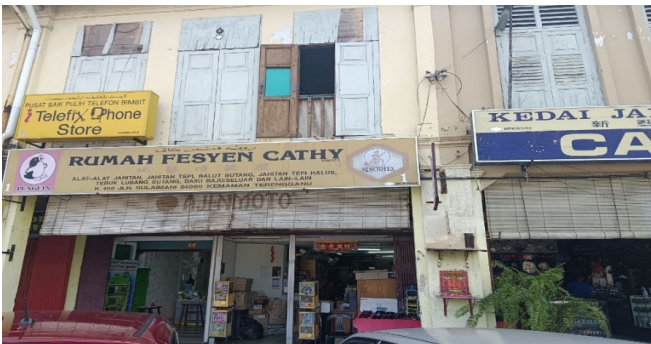
Photo 5: The window panels that have been slammed on the Jalan Sulaimani shophouse
